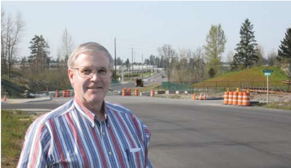
Councilmember Bush checking final construction prior to opening a new half-mile of Canyon Road between 192nd and 200th Streets.
